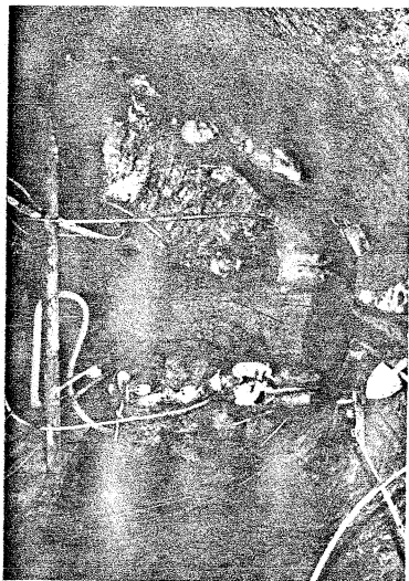
Fig. 13. Brenching out the Kaumerl pressure-shaft invert; protection by steel arches and shotcrete
