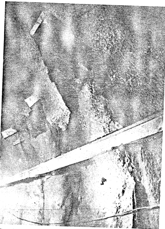
Fig. 9. Shotcrete lining failure because Perfo anchors and bottom bracing were not applied in good time
