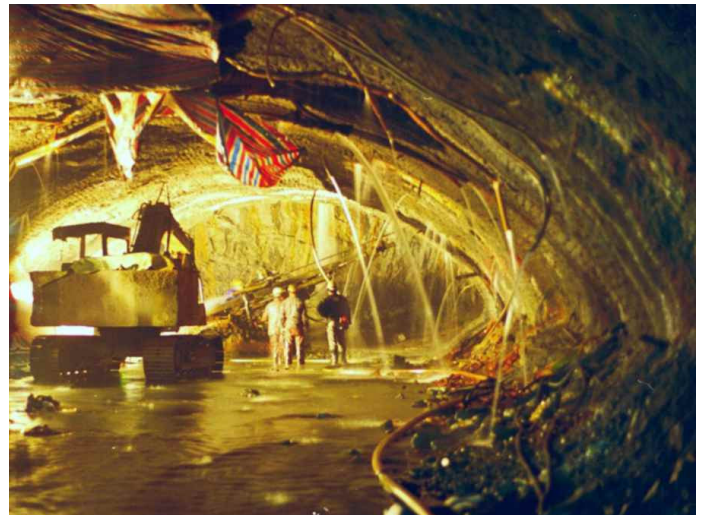
Fig. 22: The occurrence of large volumes of water can give rise to difficult construction problems in tunnels.
