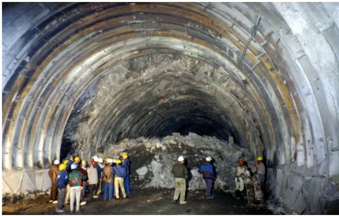
Fig. 9: Severe squeezing in a fault zone encountered by the 10 m span top heading of the headrace tunnel for the Nathpa Jhakri hydroelectric project in India.
