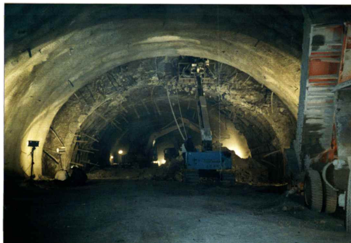
Fig. 11: Re-mining the perimeter of the 16 m span Mucha tunnel in Taiwan after severe squeezing in a fault zone. Photograph reproduced with permission from Sinotech Engineering Consultants Inc., Taipei.
