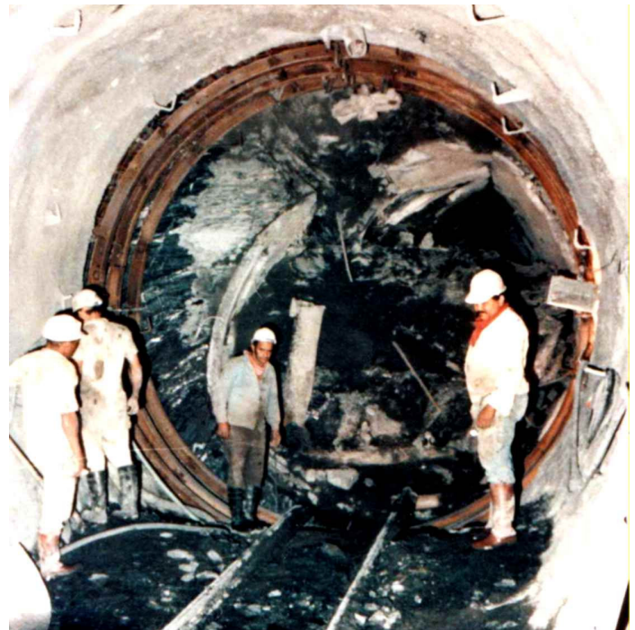
Fig. 8: Yacambú-Quibor tunnel in Venezuela. Mining out the remains of a tunnel boring machine trapped by squeezing of the tunnel during a stoppage of the drive.
