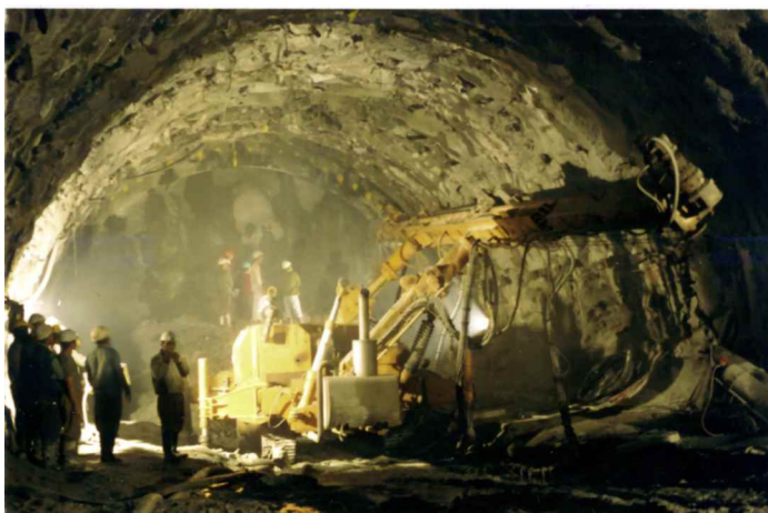
Fig. 10: Drilling unit for the installation of 12 m long 75 mm diameter pipe forepoles to form a protective umbrella under which the headrace tunnel was successfully mined through the fault zone in the Nathpa Jhakri headrace tunnel.
