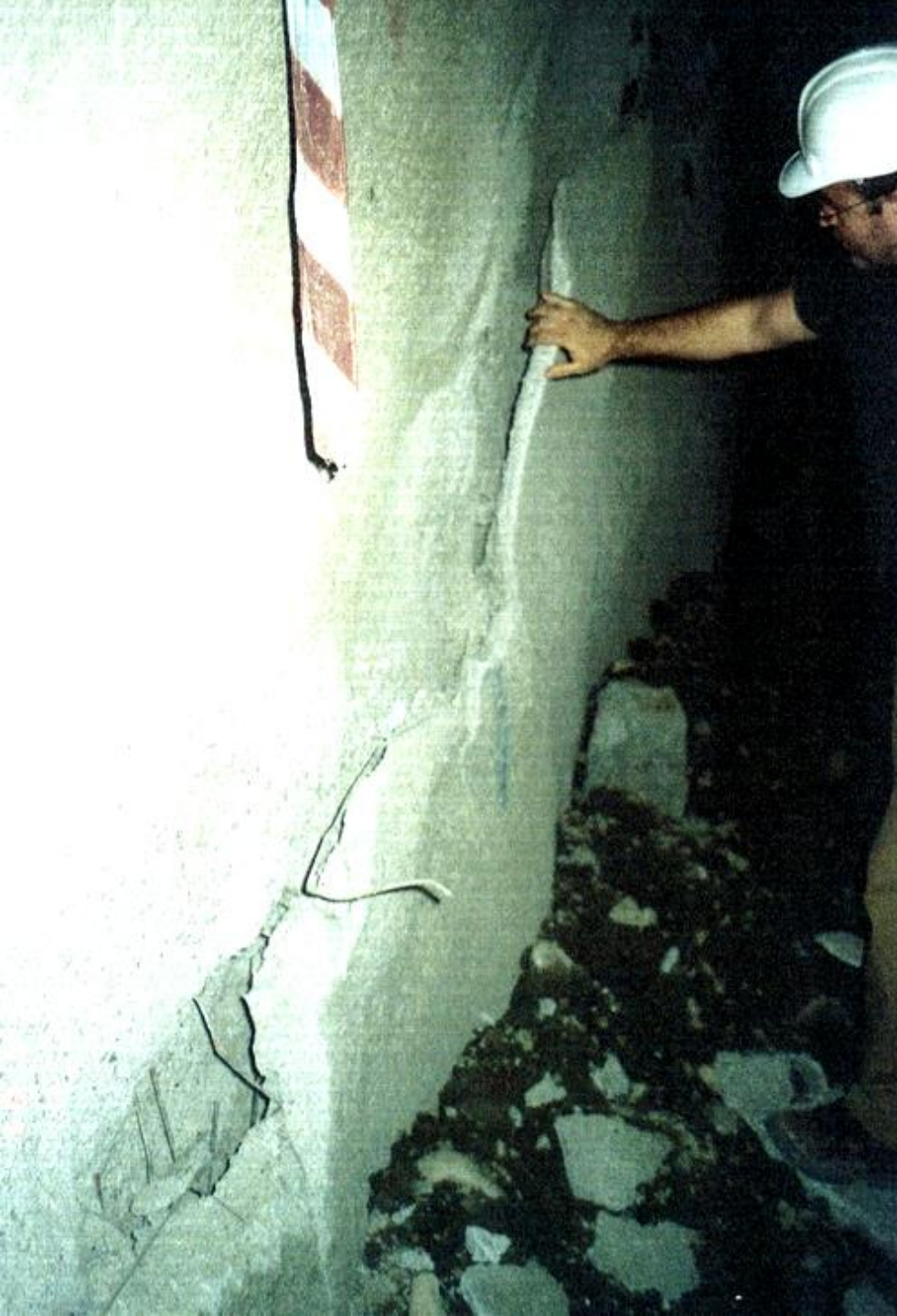
Spalling of shotcrete in the sidewall of one of the tunnels driven from the north portal of Kallidromo
