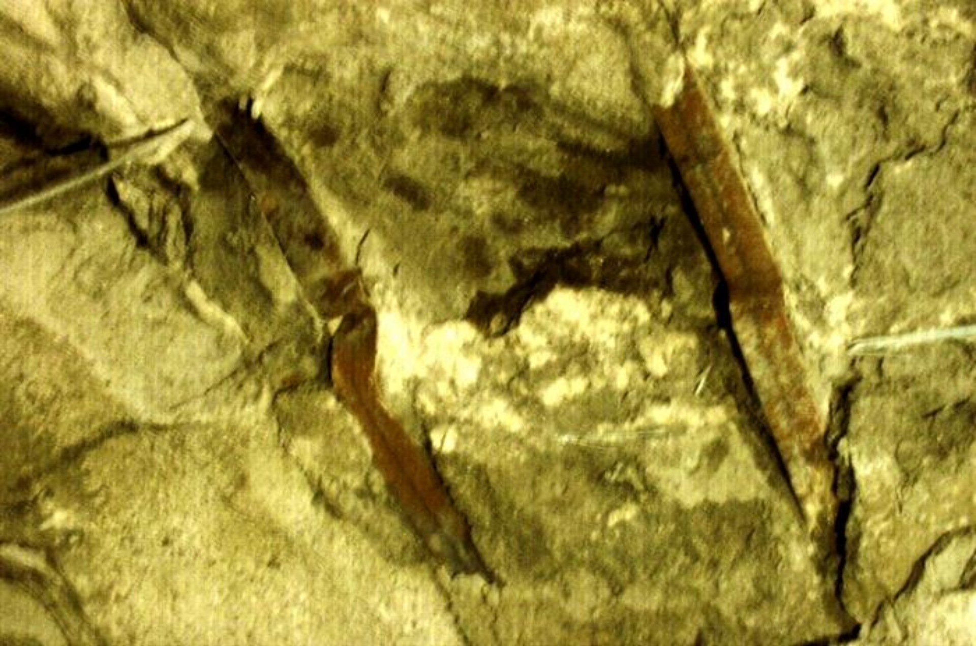
Buckling of steel sets in one of the north Kallidromo drives
