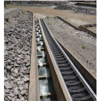
Fish ladder and small boats passage
