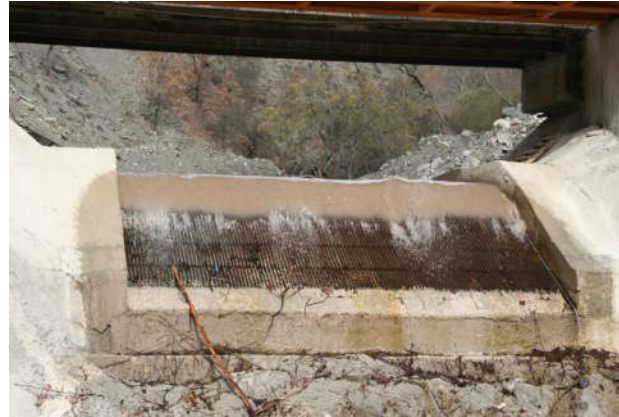
Trash rack of water intake
