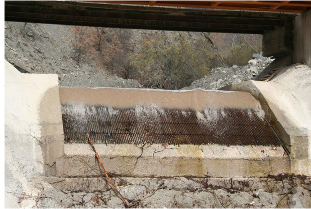
Trash rack of water intake
