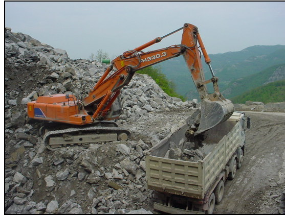
Figure 66. Rock debris of small size, mixed with dirt, is used without further process for fillings and ramp construction.
