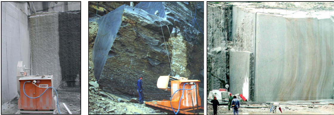
Figure 48. Examples of lateral cuts by diamond wire in different hard stones quarries. From left to right, coarse grained gneiss, gneiss and granite (Italy).
