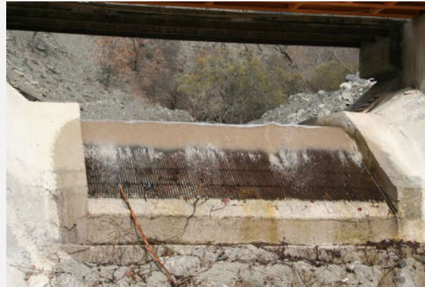
Trash rack of water intake
