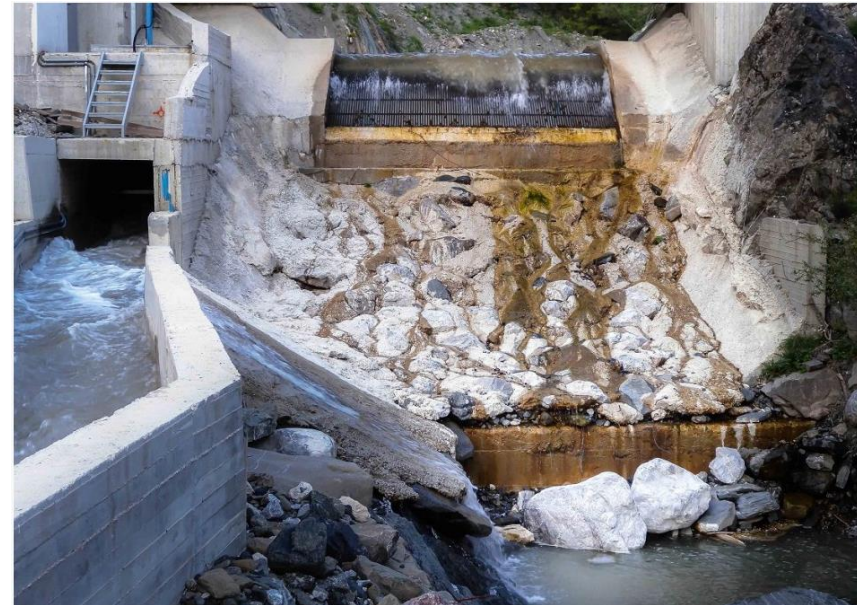
Kerasovo small hydropower plant: Tyrolean weir
