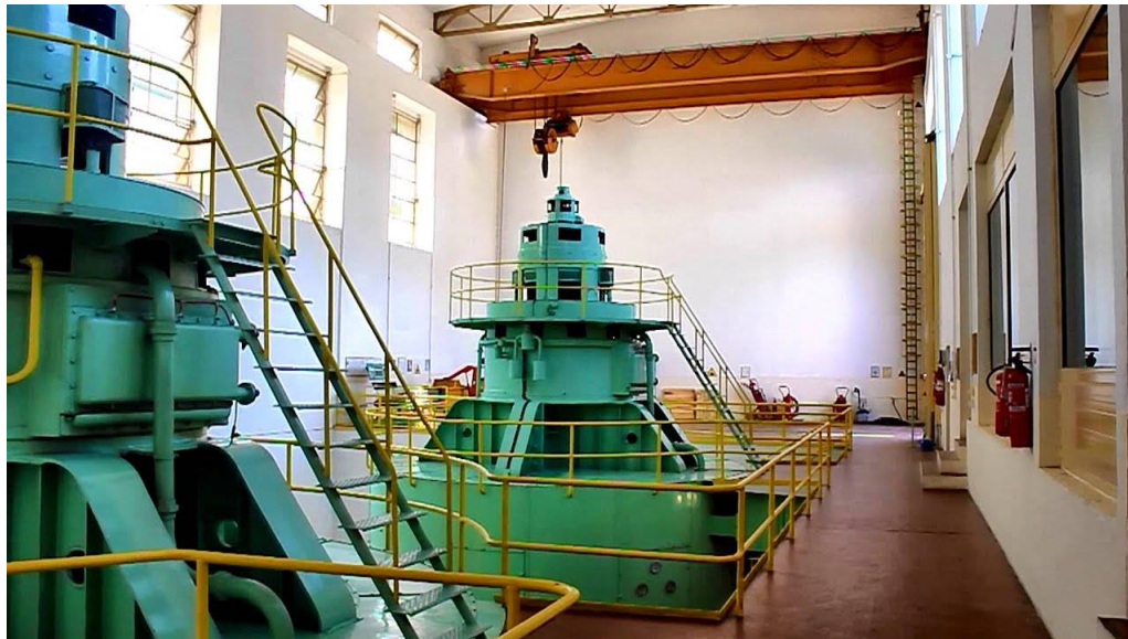
Francis turbines at Ladonas hydropower station
