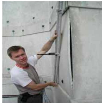
Figure 143. Thermal and moisture gradients in may give bowing of marble, regardless of the thickness
