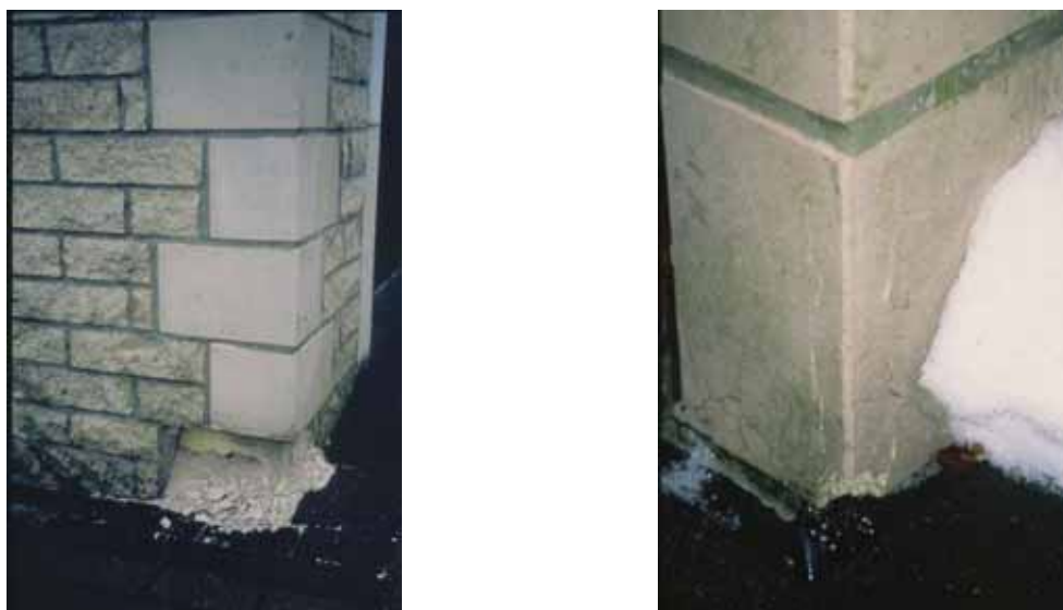
Figure 125. Quoin units in masonry destroyed by frost action
