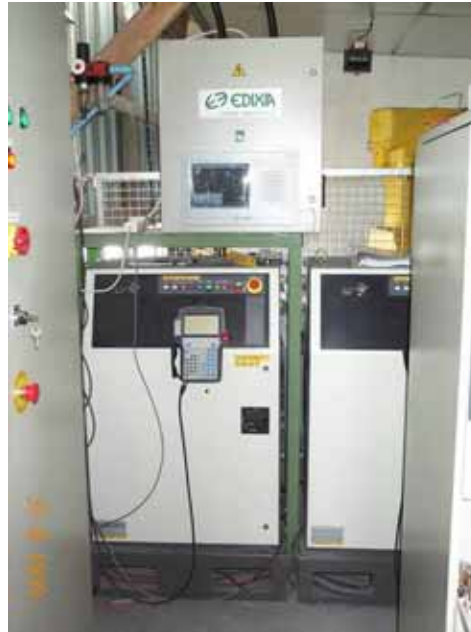
Figure 89. Example of devices that are inter-connected (PLC, artificial vision box, robots).
