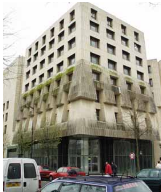
Figure 148. Formation of biological patinas on the parts of the building submitted to direct rainfall
