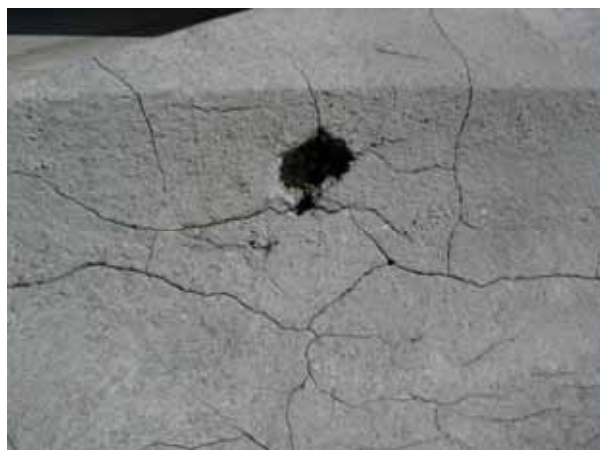
Figure 126. Pedestal of a statue cracked by the frost
