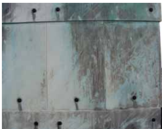
Figure 135. Discolouration of façade element due to staining from Copper studs and pollution
