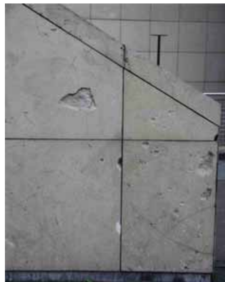
Figure 140. Splintering due to dense coating, probably due to moisture saturation behind the surface maybe in combination with frost action
