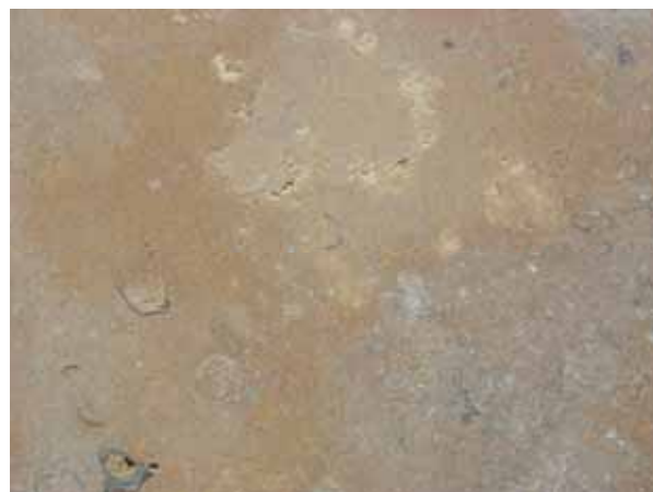
Figure 127. Beginning of scaling on a flooring slab after one winter
