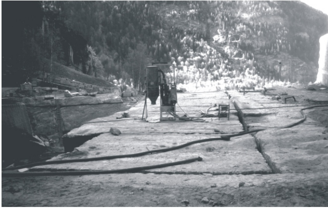
Figure 15. A primary block has just been loosened by blasting, and moved approximately 10 cm. Serizzo quarry, Italy.
