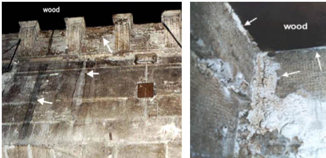
Figure 29 Example of an interaction between wood and rock in a building. Coatings from wood provide a higher pH, humidity concentration and reactions in contact.
