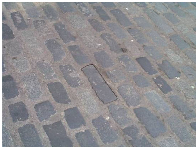
Figure 26. Shear failure of a single sett
